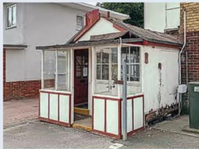
A front view of the old Skegness railway coal office being dismantled in Lansdown Road for renovation and re-erection at the new South Loop station on the Lincolnshire Coast Light Railway; the clerestory roof has already been removed. DAVE ENEFER/LCLR
