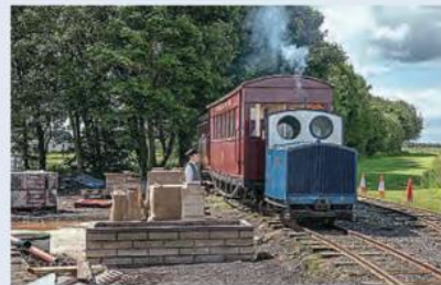
Construction of the new station is well underway, with Motor rail Simplex 4wDM No. 3995 of 1926 Paul in the platform road with a passenger service for Walls Lane, consisting of former Ashover Light Railway and the 'Queen Mary' ex-Nocton Estates Railway carriages. The combined age of the trio is about 300 years! DAVE ENEFER/LCLR
