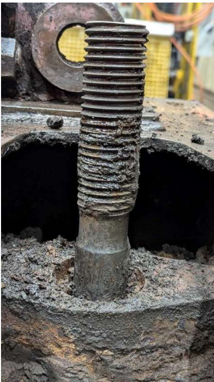
Picture 23 – Spring Hanger Stuck Solid
