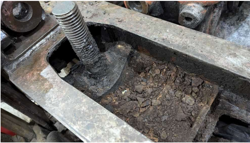
Picture 24 – Spring Hanger Stuck Solid
